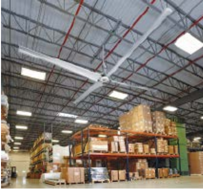
HVLS fans help HVAC systems work efficiently.
