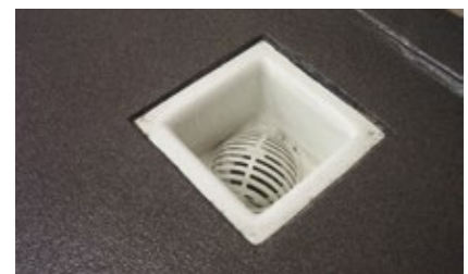
A certified coatings professional may recommend converting trench drains into box drains (shown) to reduce the wet surface area available to trap bacteria.
