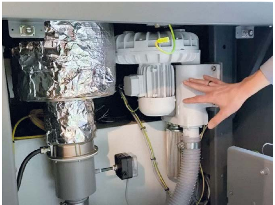
Figure 2: Leister electric air heater blower installation on large roasting machine.
