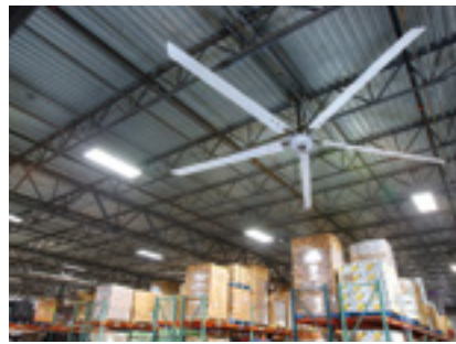
HVLS fans, like from Hunter Industrial, can help increase indoor air flow to previously underserved areas.
